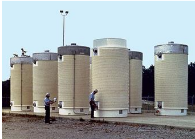
Figure 4.1 Vertical Casks on a Concrete Pad Being Monitored xiii
